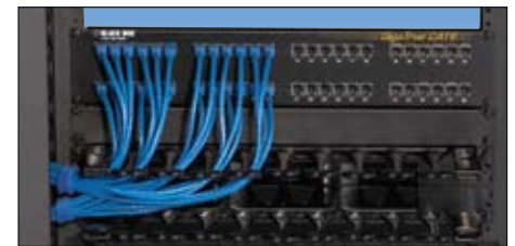
Horizontal Cable Managers keep patch cables organized.
